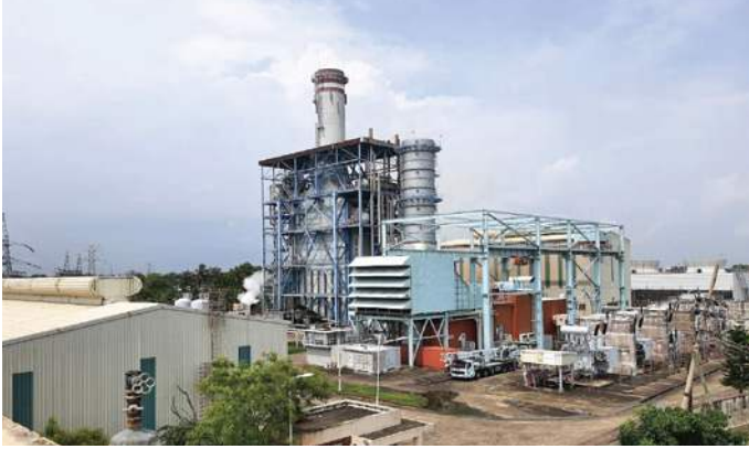
Chandpur 150MW Combined Cycle Power Plant
